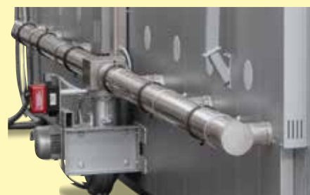
Cooling system with fresh air fan
